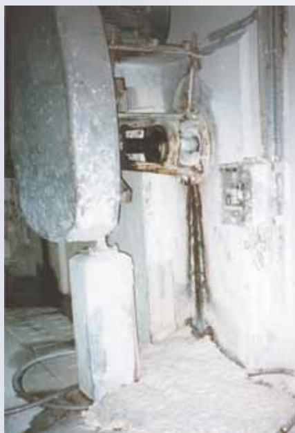
Soiling and product loss: Accumulated leakage at a side-driven chest agitator sealed with a packing.
